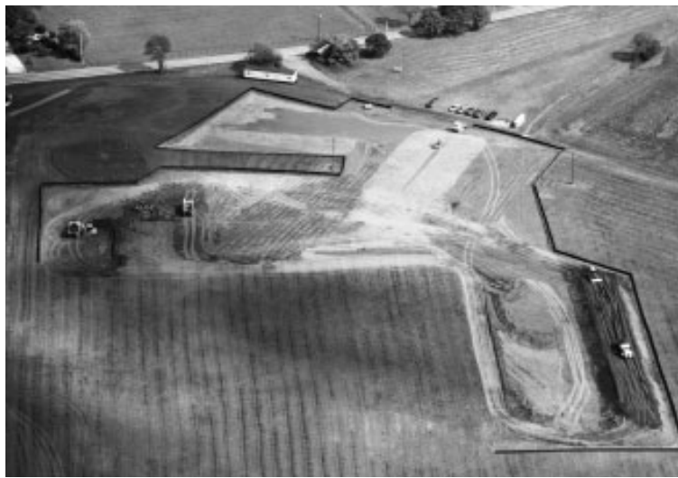
As seen in this aerial photograph, work has begun on Constellation Energy's 100-acre solar power system.
