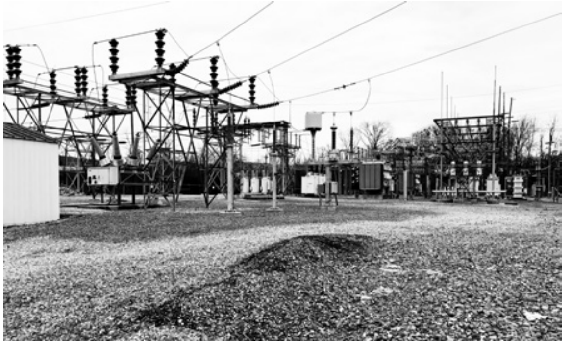
Electrical Substation where the Thurmont power grid is connected to Potomac Edison's distribution system. The Thurmont Town run power systems dates back to the early 1920s when there was no state or national power grid and every town was on its own.
